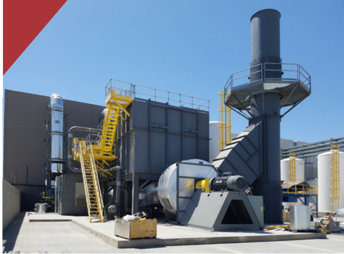
70,000 scfm RTO (Can Coating Application)
